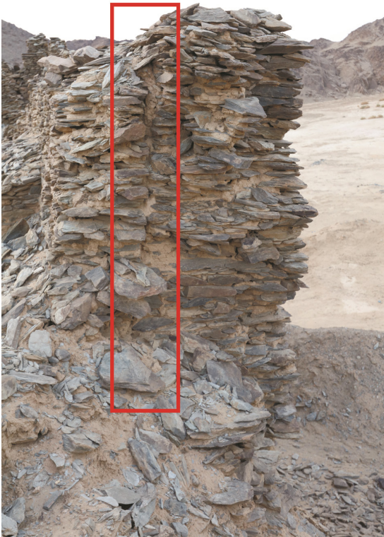
Figure 4. Absence of masonry connection facing along the northeastern wall. Photo: D. Fedorova
